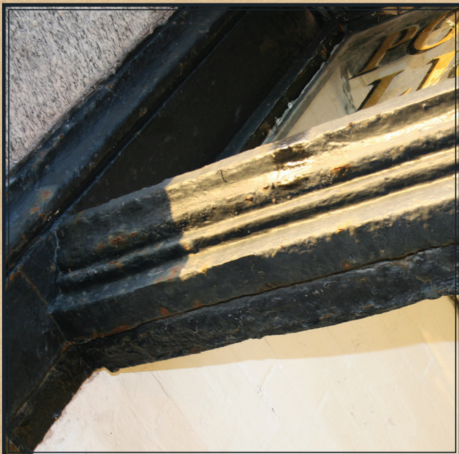
Tower main entrance cast iron door frame before restoration; collection of the Ponce De Leon Inlet Lighthouse Preservation Association
