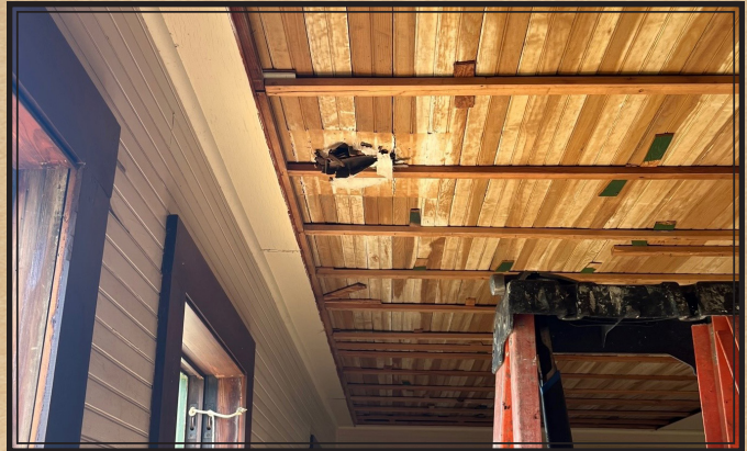
Restoration work inside the Pacetti Hotel dining hall revealed historic beadboard above modern 4'x8' ceiling panels
