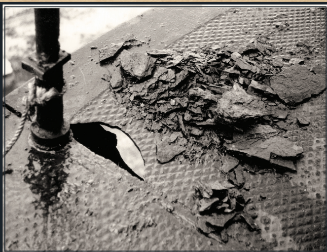
Visible deterioration of the tower gallery deck in 1972; collection of the Ponce De Leon Inlet Lighthouse Preservation Association
